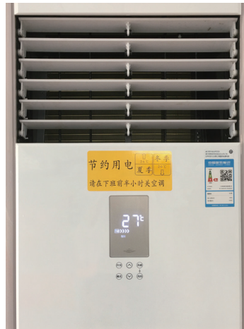
Air Conditioning Temperature Control
